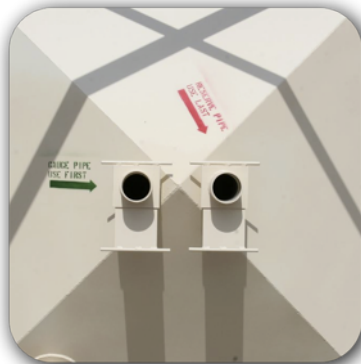
4" Filler Pipe and 4" Reserve Pipe
